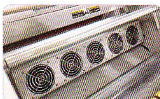
Air cooling system
